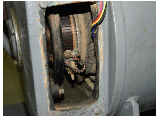
Fig 7: The temperature sensor inside the motor
